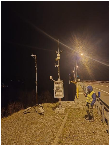
Fig. 1. Field deployment near a motorway tunnel portal with two WindSonic ultrasonic anemometers installed at different heights.
